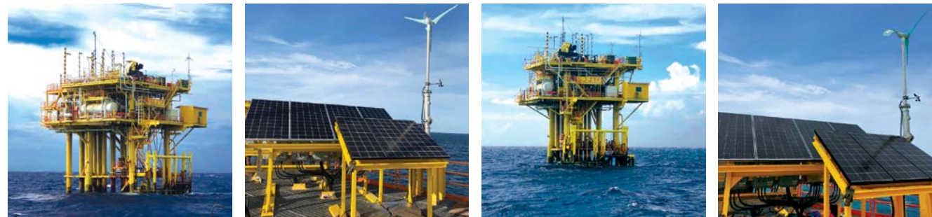
Wind Turbine Solar Hybrid Installation at SFJT-F (two units).
